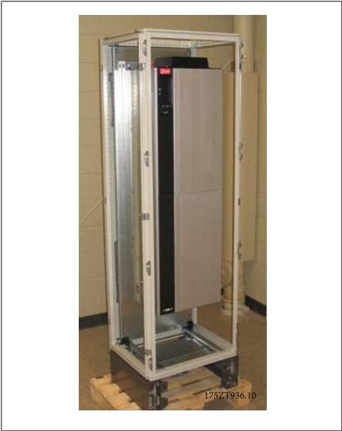
Illustration 3.36: Frequency converter installed in cabinet
